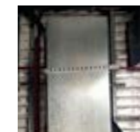
Air Vent and Ducting Reference Officeworks ceiling Photograph taken by Tyler Hill
